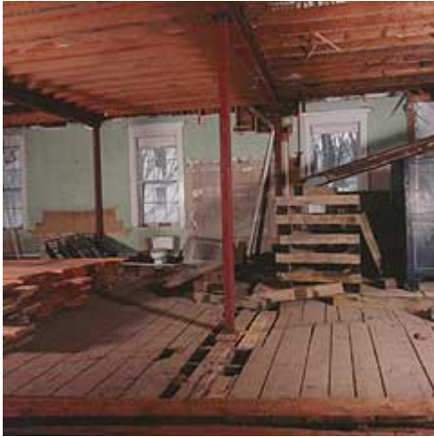
Figure 2: Floorboards removed from the first floor in Nantucket Atheneum
